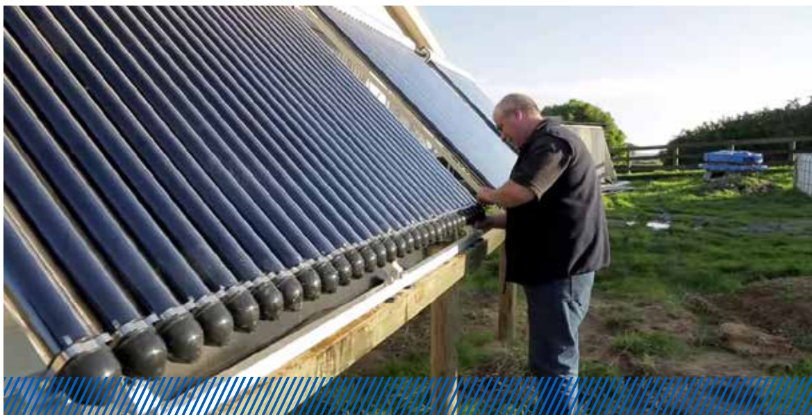
New solar hot water systems are softening the impact of King Island dairy farmers on the environment.
